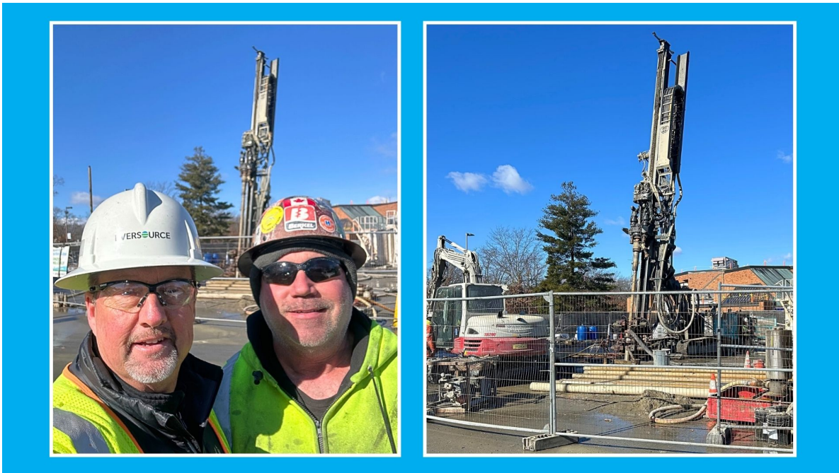
Eversource Construction Manager Matthew Knowles (L) celebrates the drilling of the final borehole with Berkel drill team at Farley Lot – Feb. 2024
