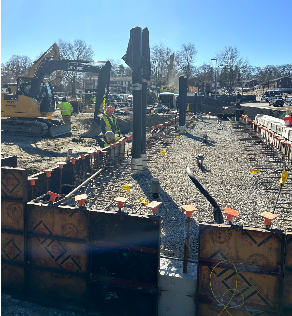
RH White continues with piping at the pump house in the Farley Lot – Feb. 20, 2024
