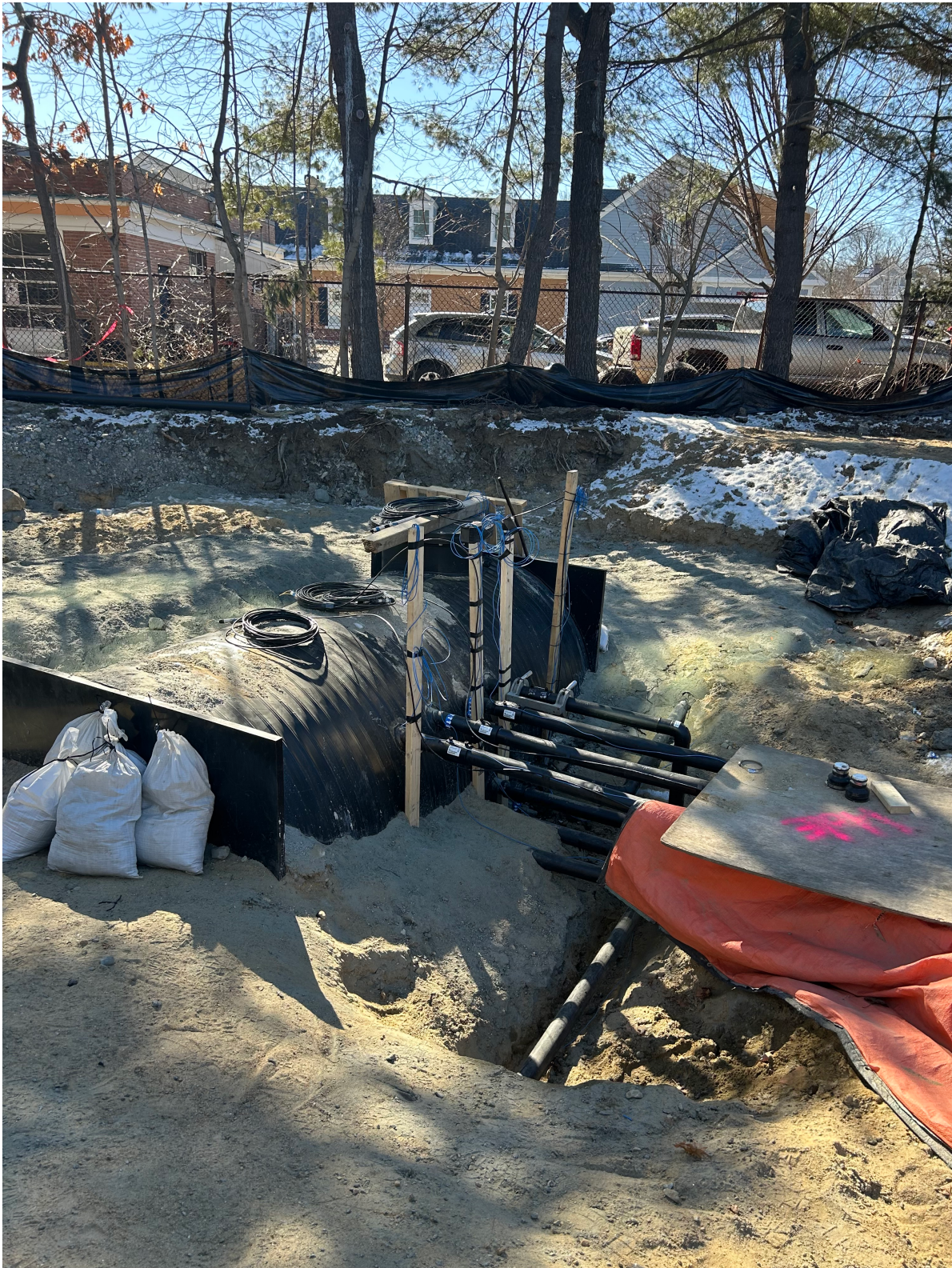
Framingham Fire Station - RH White crews continue to run and test the piping of the loops and main runs – February 20, 2024
