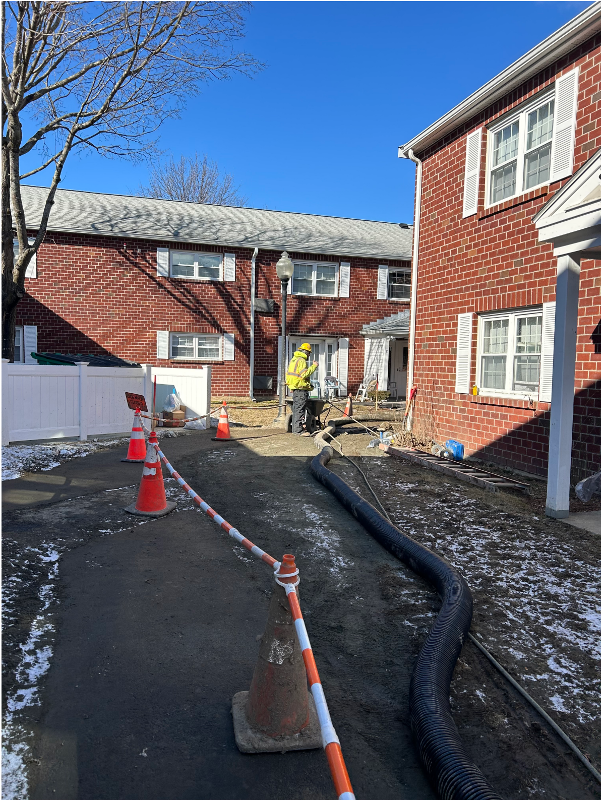
Crew on John J. Brady Ln. installs service piping in between FHA buildings – Feb. 16, 2024
