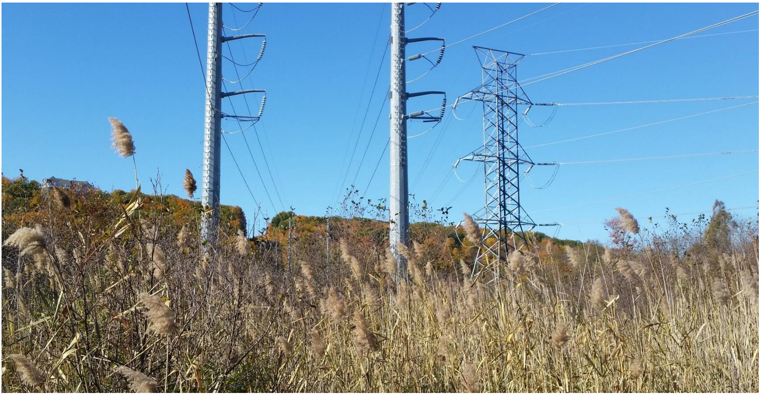
Photo #1: View of Wetland W-1 from the west side of the Plumtree Substation. Existing 321 Line Structure 10269 is shown on the right. Facing West.
